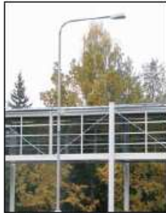
Base station integrated into lightpole
