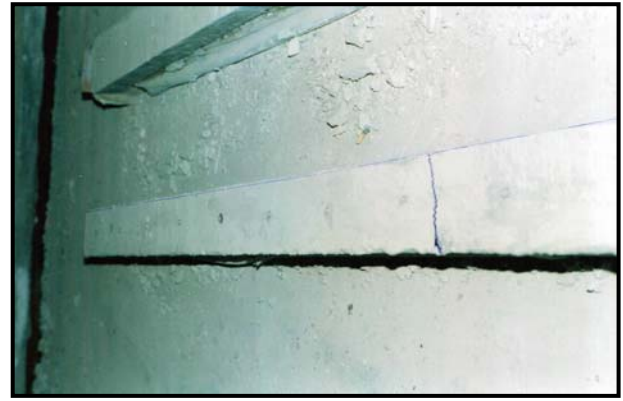
Plate (4.2) : The Crack Location in Specimen (SM 2.5 )
