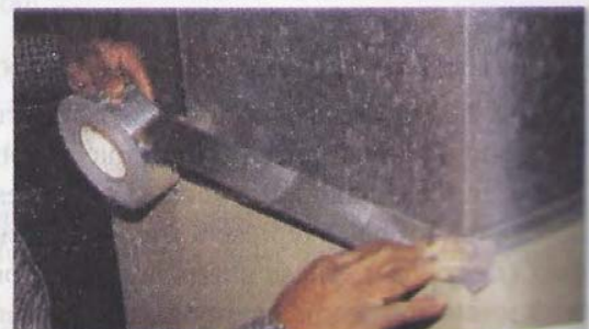
Taped duct connection.
