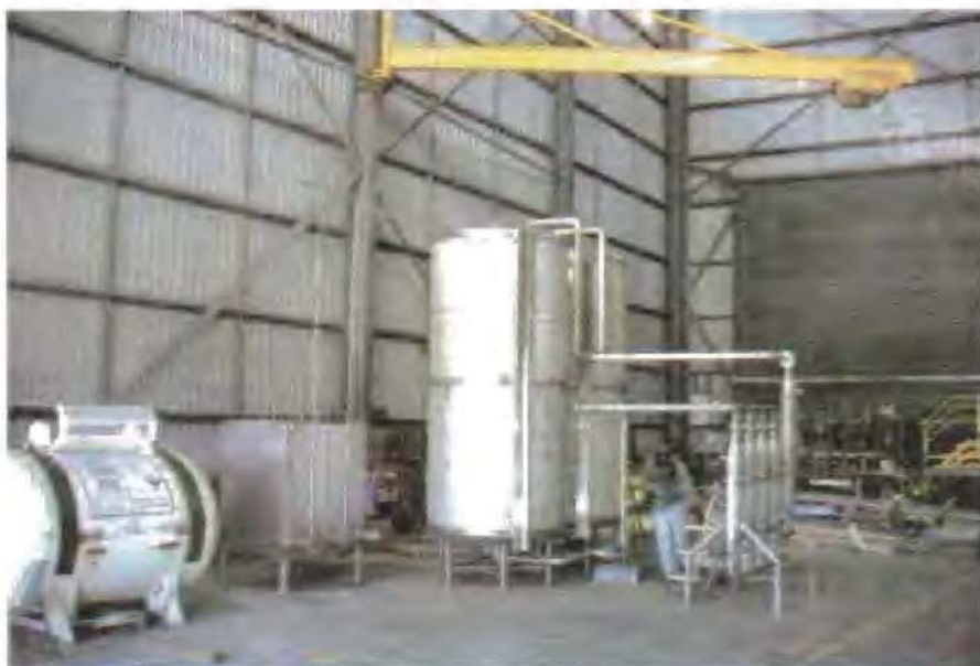
Ammonia refrigeration plant.
